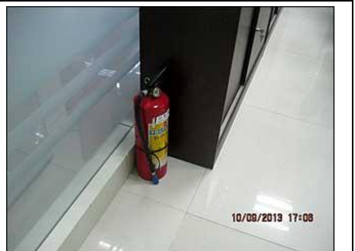
Extinguisher in office,
