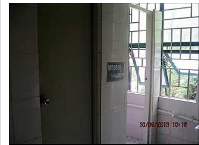
Toilets provided with appropriate privacy
