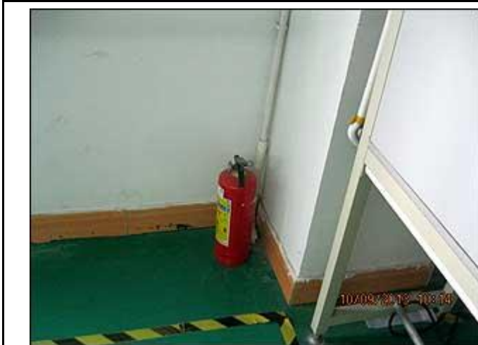
Extinguisher in factory,
