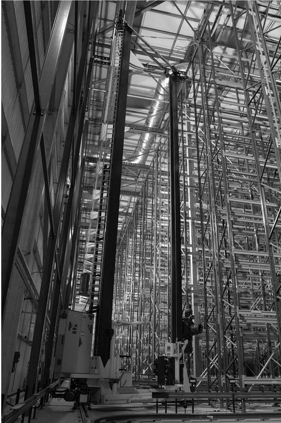
Figure 16.8 AS/RS aisle-changing crane (courtesy of FKI Logistex)
